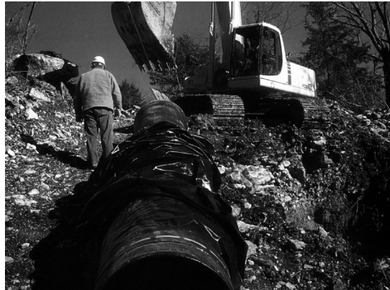
The versatile performance capabilities of AMERICAN Flex-Ring Joint Pipe are perfectly suited for projects containing a variety of conditions such as the hilly, rocky terrain shown in this photo.
