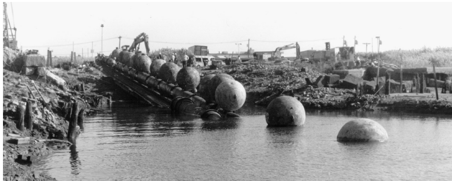
Flotation provided by attached spheres facilitated installation of this 30" pipeline with Flex-Lok Joints.
